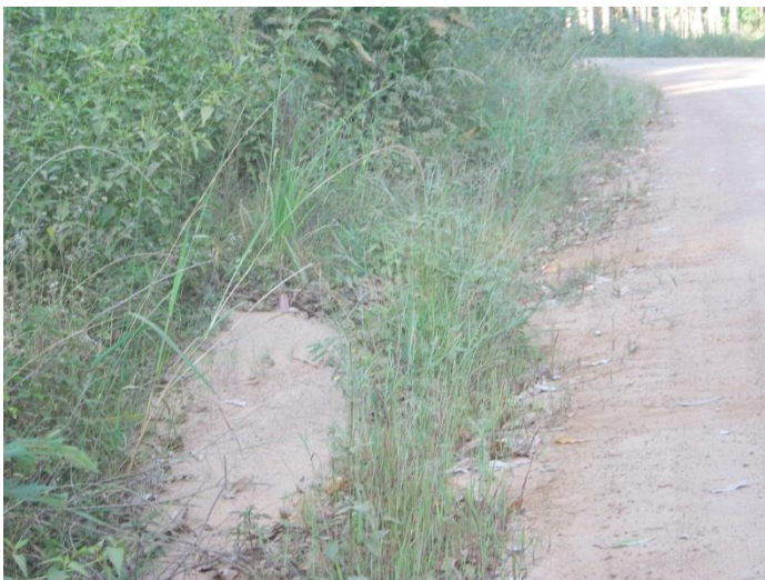
Fig. 4: Over-grown and silted side drains
