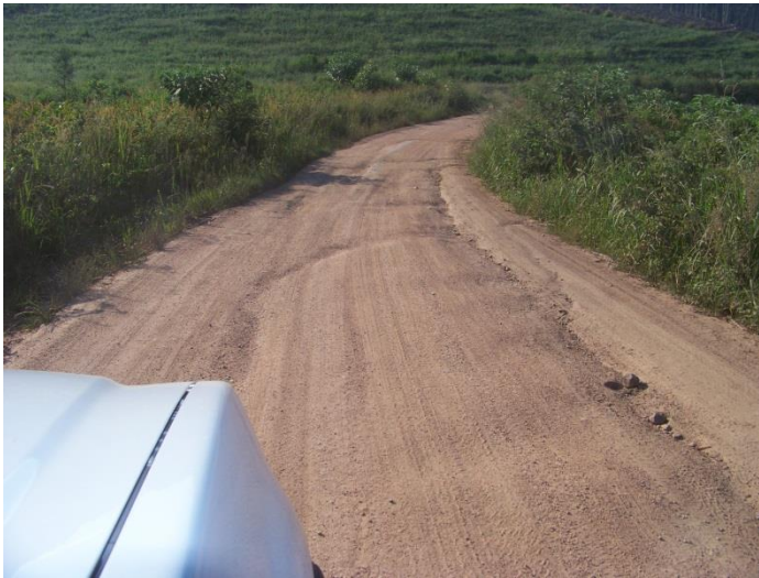
Fig. 5: Formation of erosion channels
