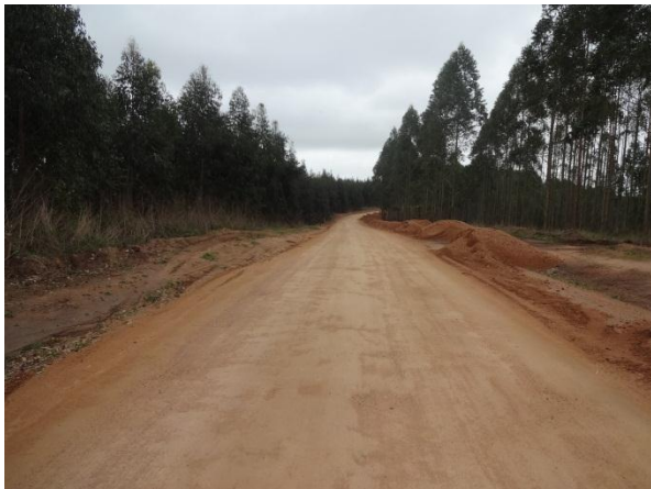
Picture 5: Taken from the gravel surface condition of the road to be upgraded.
