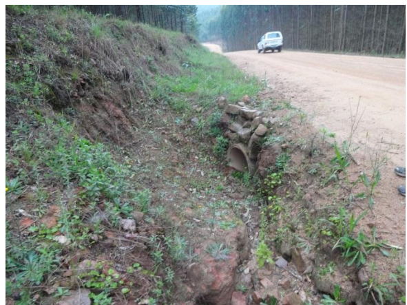
Picture 10: Pipe culvert without outlet causing erosion to adjacent properties.
